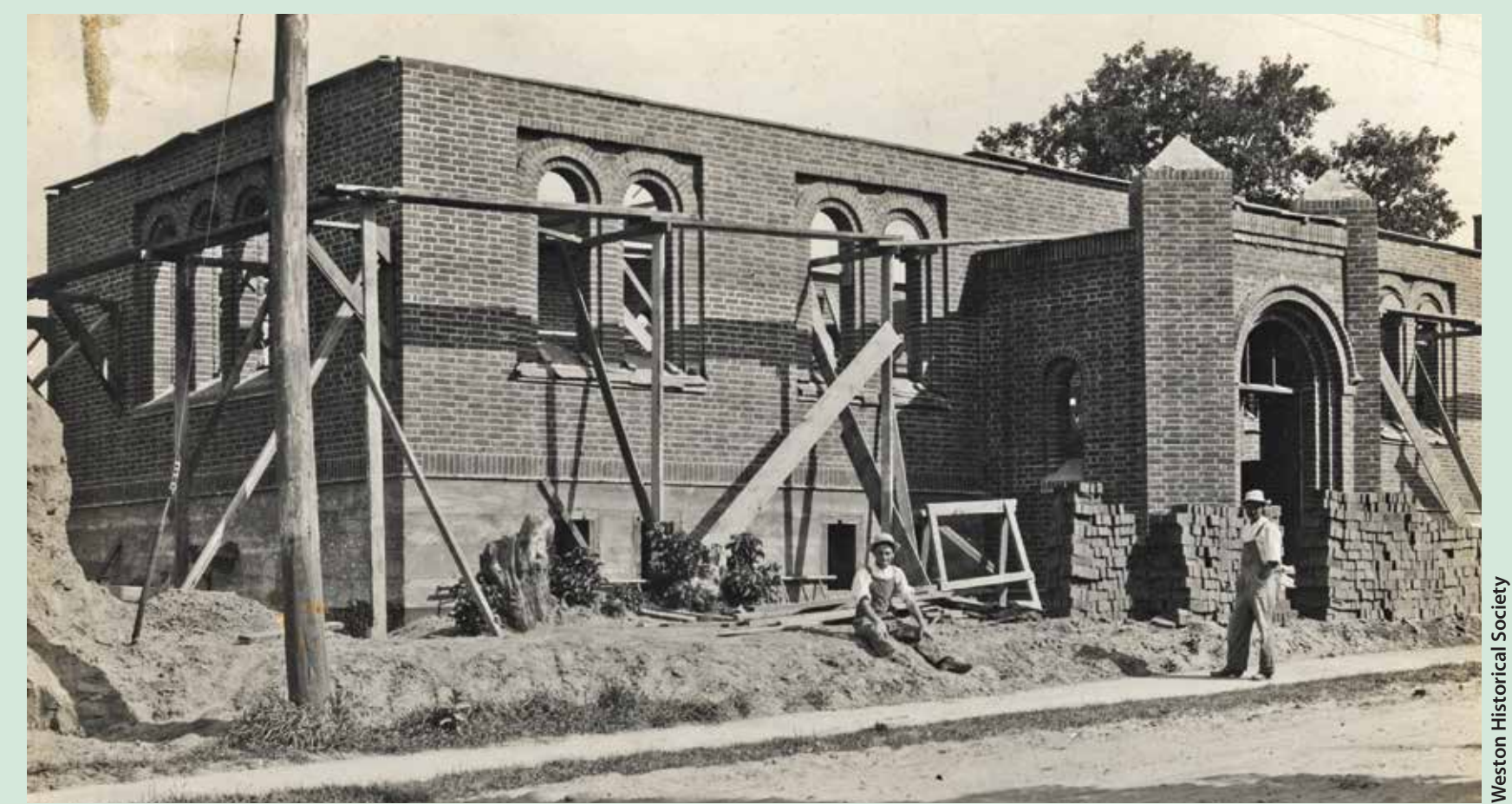
Construction of Weston Public Library, summer 1914 George Sainsbury (1875-1951), a Weston contractor and builder, started excavation for the library on April 8, 1914. By July 10, the walls were almost ready for the roof. Sainsbury, who also was on Weston Council in 1913 and 1914, was paid $7,445 for his work.
